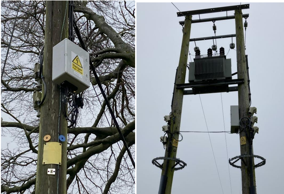
Figure 8 Location of installation of Polesight device on a single pole and on a H Pole, showing the Rogowski coils measuring the second feeder
