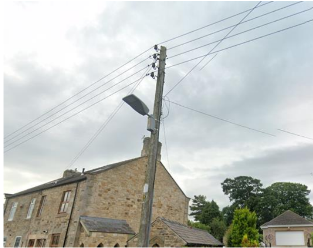
Figure 31 Location 1 – Pole outside West House
